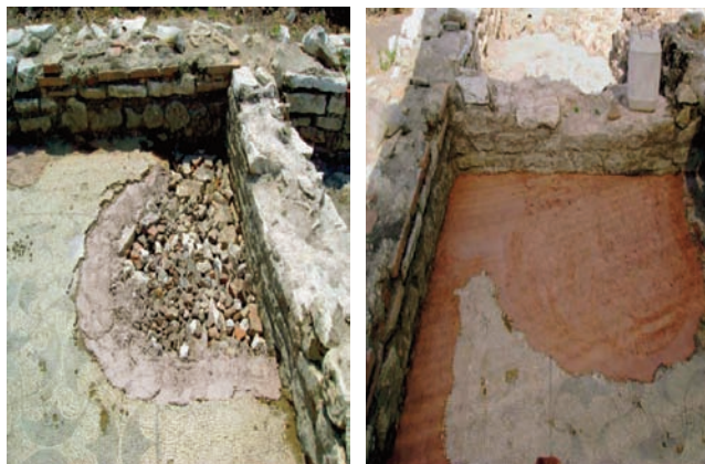
Building up permeable layers of stones and tiles in lacunae in the Vrina Plain mosaic prior to capping with lime mortar.
