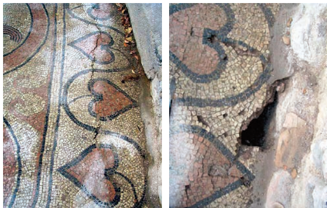
Active cracks and new lacunae in the Baptistery mosaic pavement.
